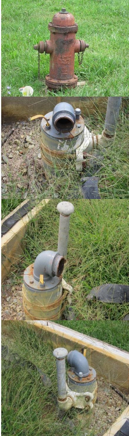
Abandoned fire hydrants and wells in Old Town Cheswold
